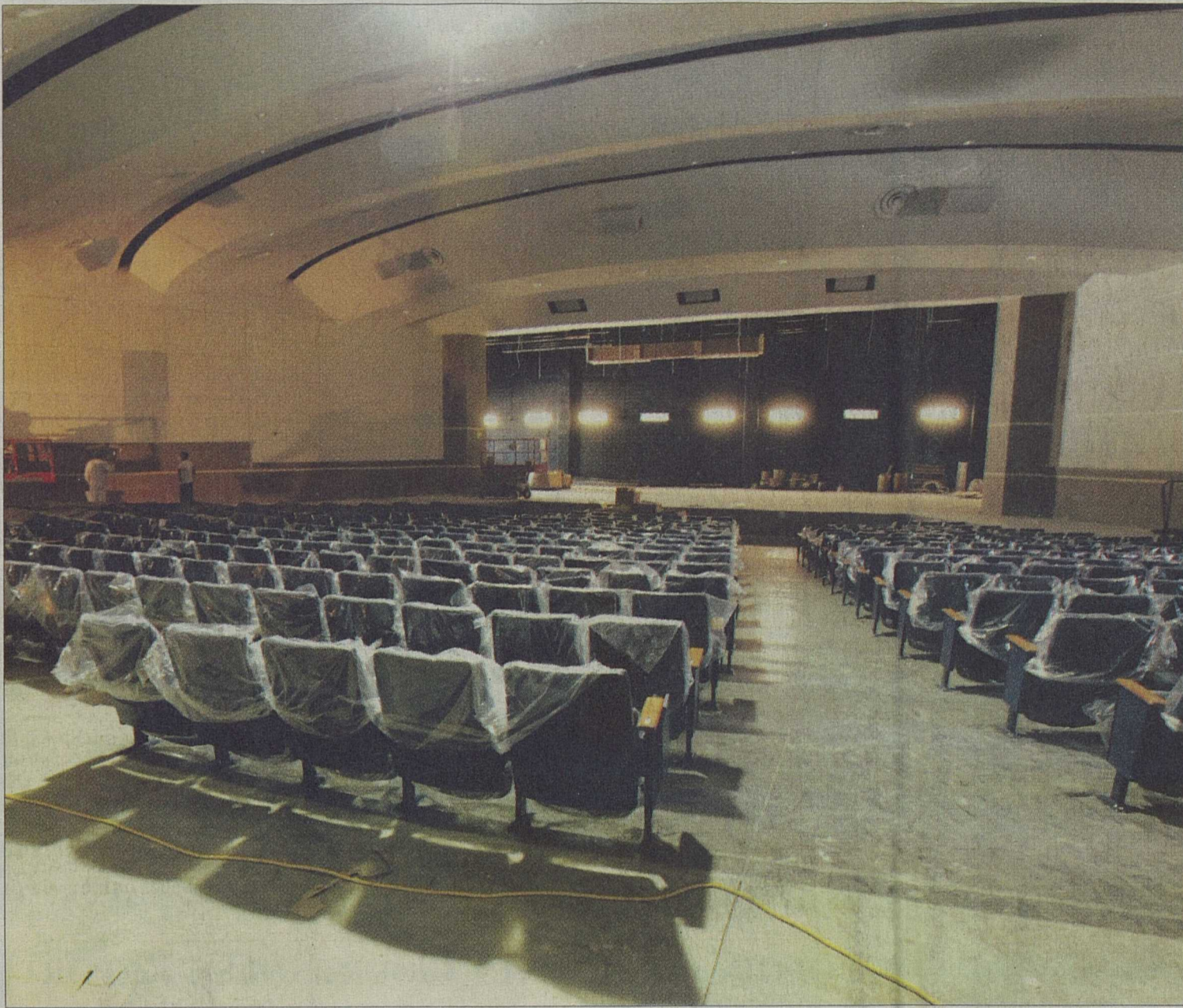
The Rice High School Auditorium is taking shape in Altair. Construction of the new facilities is due to be completed in July.
